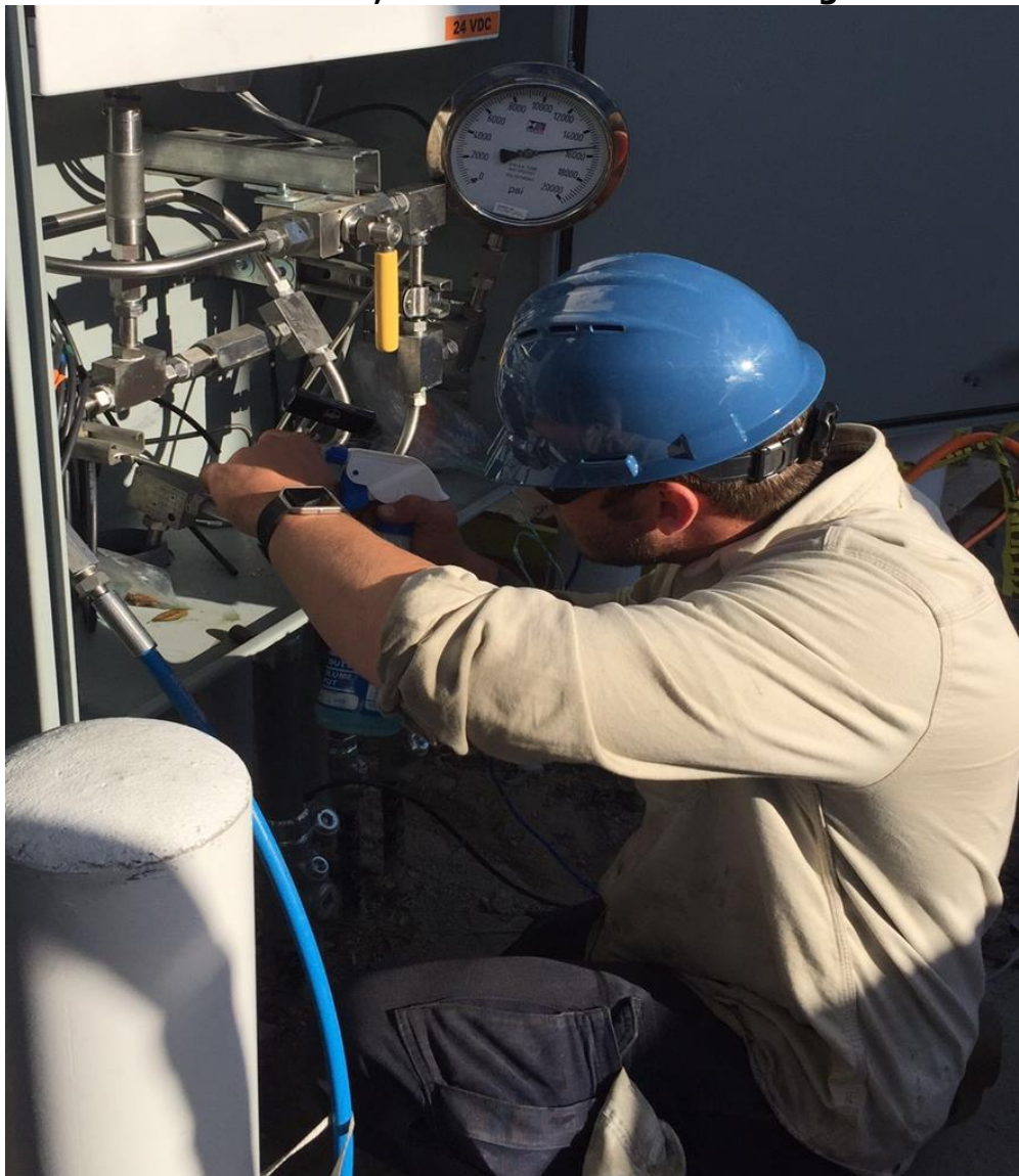
Figure 6: FirstElement Fuel, Inc. Technician Performing Pressure Check
